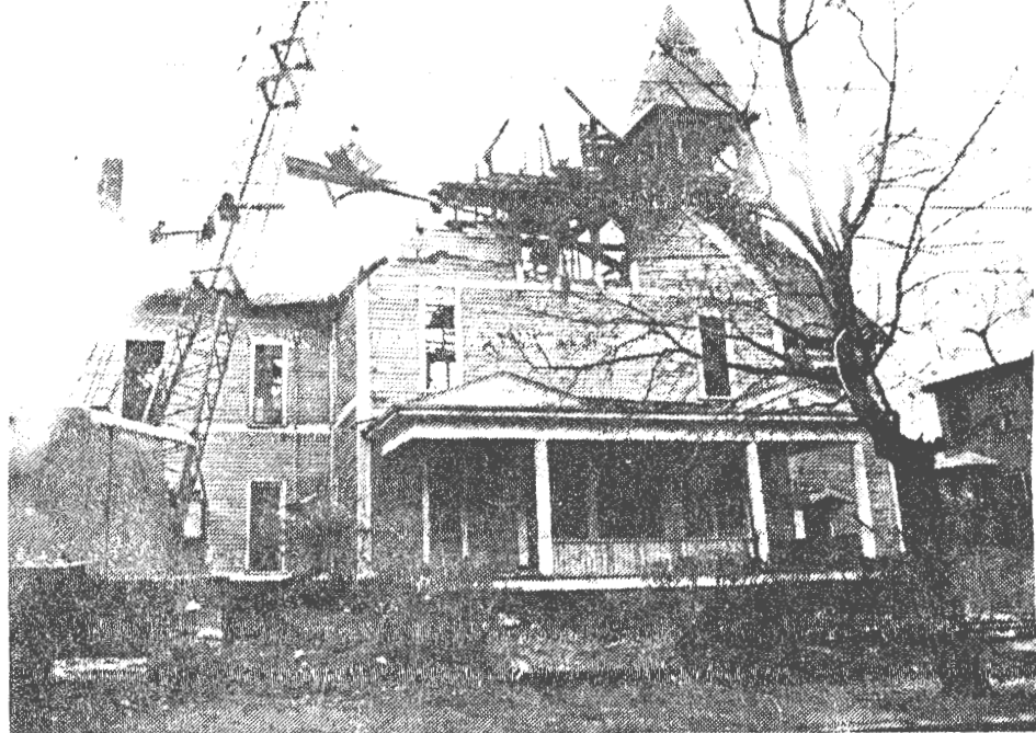
WRECKER'S CRANE demolishes the fire-damaged Linden Congregational Church building on Lawrence St., which housed Project Triangle after it was closed as a house of worship. The church bell has been donated to St. Luke's Episcopal Church. (Photo by Tom Hiltz)
